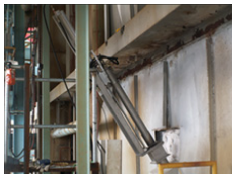
Installation complete – with cover removed
